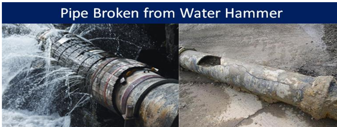
Figure 2 – Damaged Pipes from Water Hammer Effect
